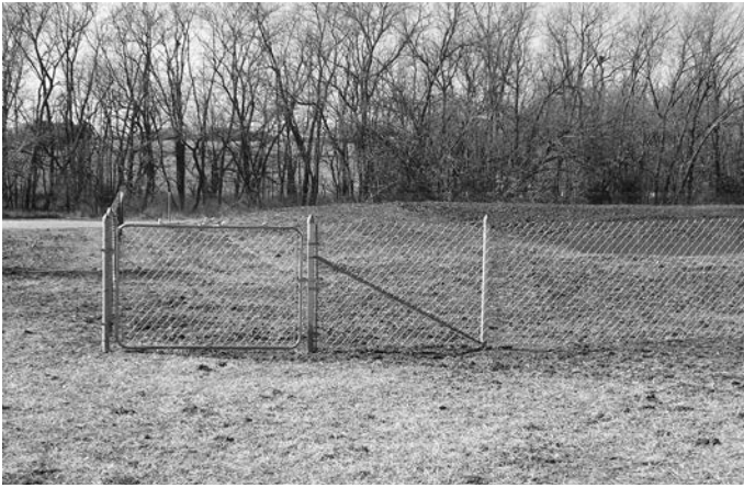
Figure 1. A lagoon with a good fence and gate outside the toe of the embankment.
